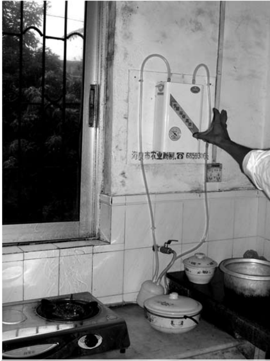
A typical biogas installation in a household kitchen. © Ben Greenhouse
