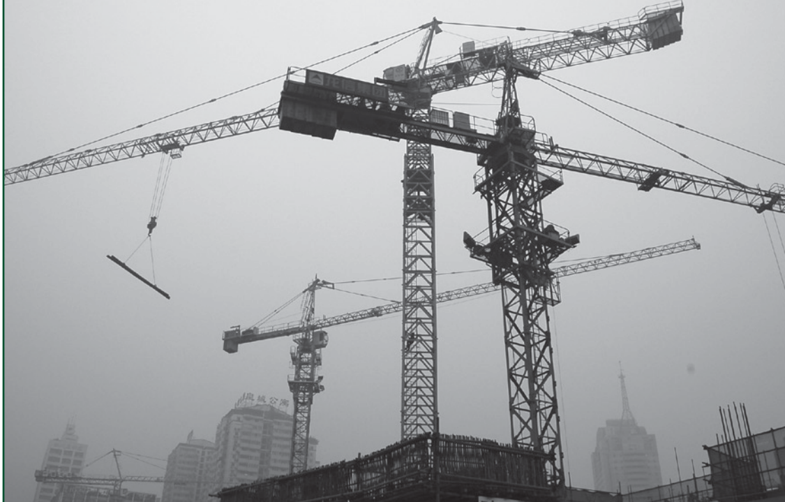
In June 2008, Beijing authorities ordered a two-month ban on construction in the city to help guarantee cleaner air for the summer Olympic Games in August 2008. Photo Credit: Andrew Chang
